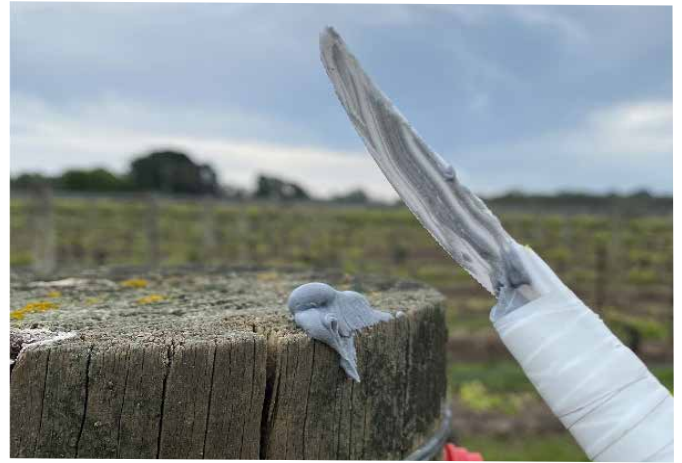
Figure 5: Application of SPLAT to the tops of intermediate posts via a caulking gun [Photo: Neil Hinchey].
